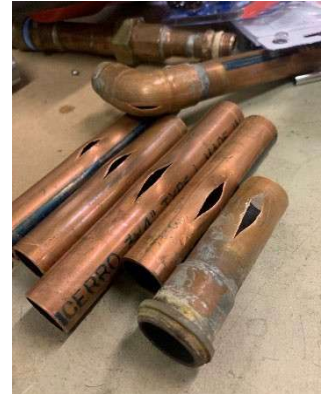
(above: burst pipes)
