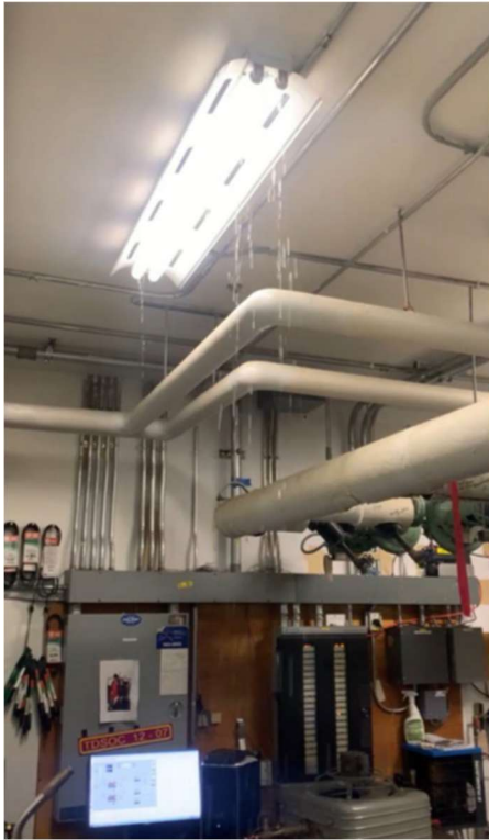
(above: water pouring through the light fixture at NSRL)
